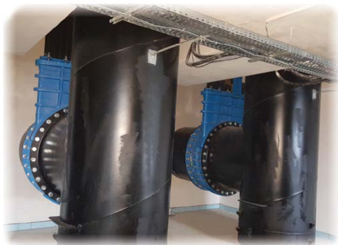
Series 200 clean water treatment application
