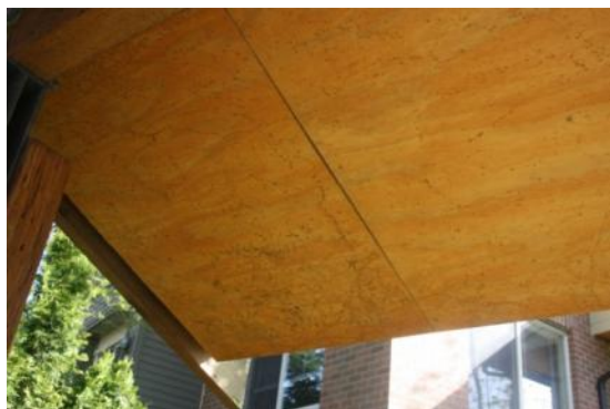
Photo 1: mold growth on the plywood cover below the sensor locations for the control roof assembly. This mold growth is after two winters exposed to ambient conditions at the study location.
