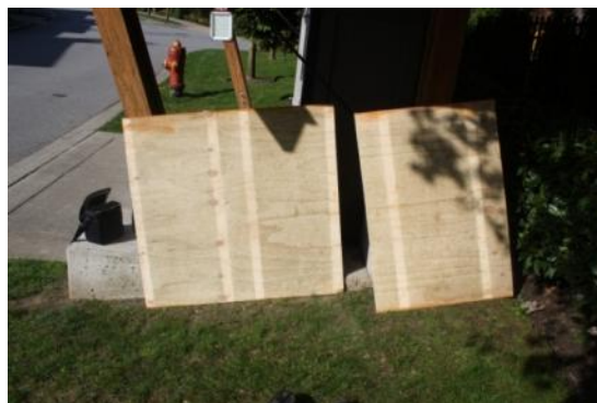
Photo 2: staining of the backside of the plywood cover. Notice at the location where the plywood was in contact with the rafters is clean.
