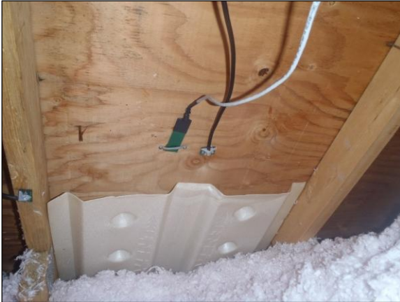
Figure B.25: Unit 4 north baffle
