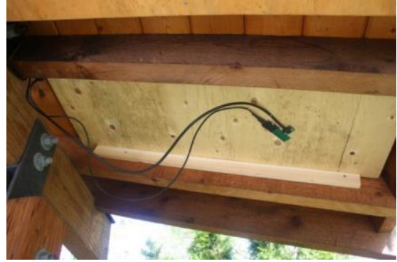
Photo 4: Mold growth on the plywood sample that is decoupled from the asphalt singles by a thick wood deck and 25 mm extruded polystyrene insulation.
