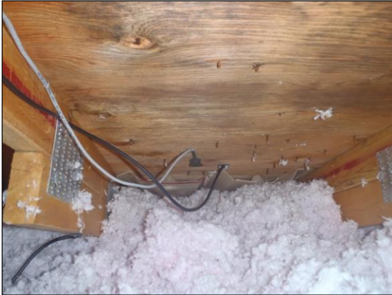
Figure B.1: Unit 1 east baffle
