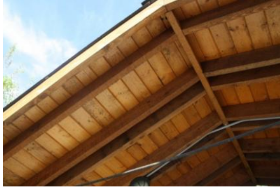
Photo 3: Mold growth on wood rafters and tongue and groove wood deck.
